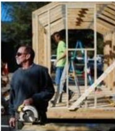
Volunteers construct a functional tiny house during the Alachua County Affordable Housing Summit on Tuesday at the Alachua County Health Department. — Rob C. Witzel/The Gainesville Sun
